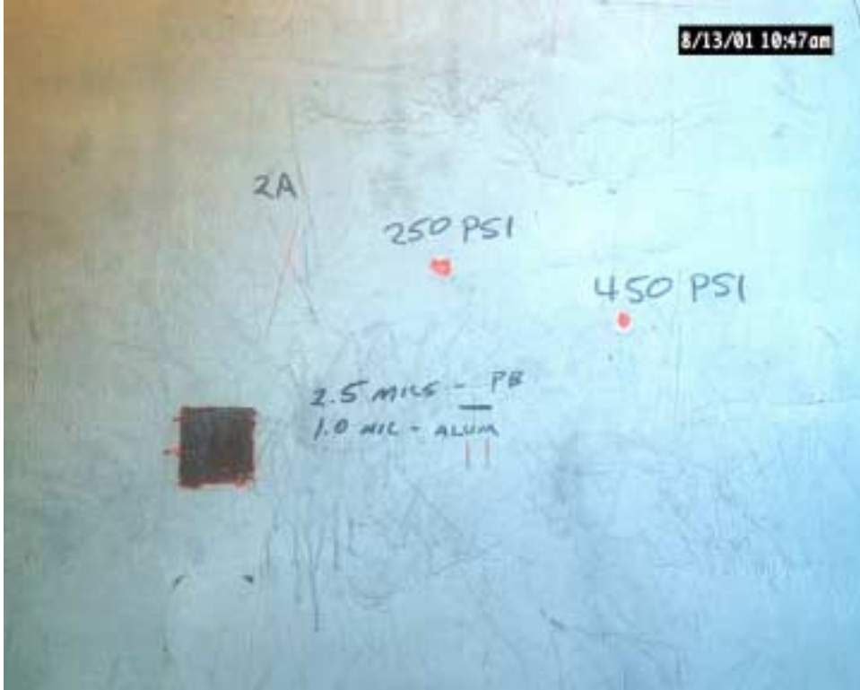
Figure 17. Test area on the KY 551 Bridge in Adair Co. showing tensile adhesion results, knifing adhesion results, and Tooke coating thickness readings.
