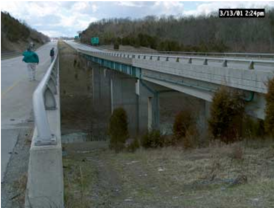
Figure 10. KY 9002 (Bluegrass Parkway) over Chaplin River in Washington County prior to painting.
