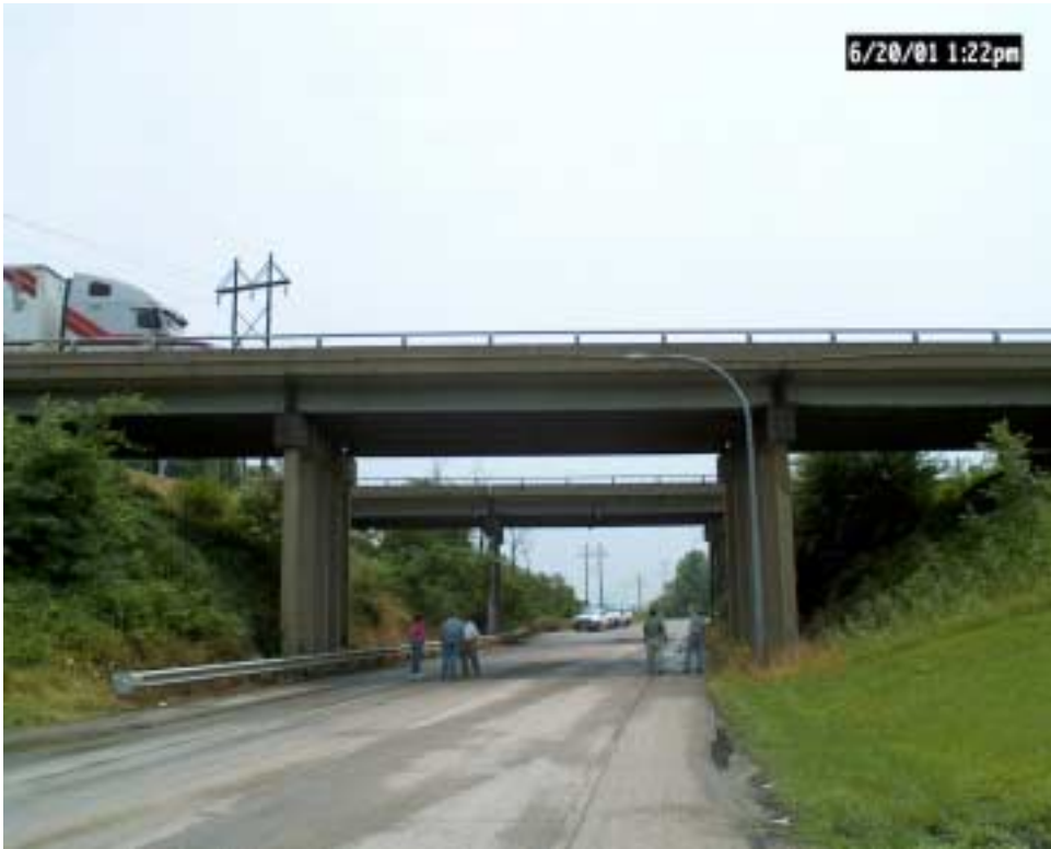
Figure 11. US 60 bridges over the CSX spur in Daviess County prior to painting.
