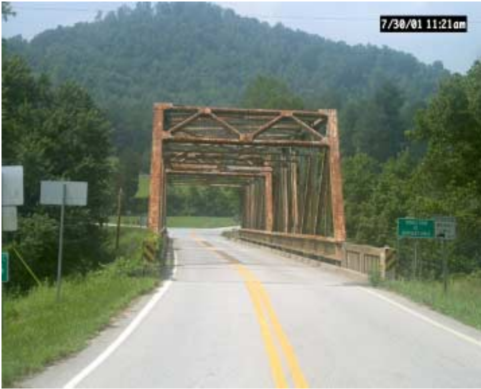
Figure 5. KY 30 over Middle Fork of the Kentucky River in Breathitt County prior to painting.
