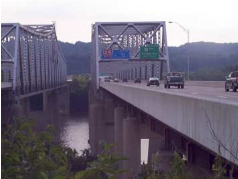
Figure 6. I 275 twin bridges (Combs-Heil) over the Ohio River in Campbell County prior to painting.
