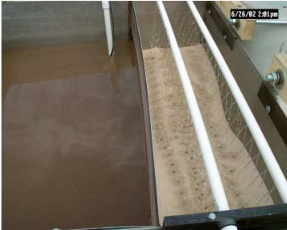
Figure 41. The wastewater holding tank and the sand bed of the filter system.
