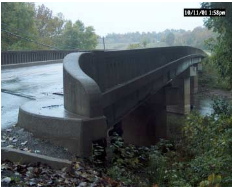
Figure 12. KY 139 bridge over the Little River in Trigg County prior to painting
