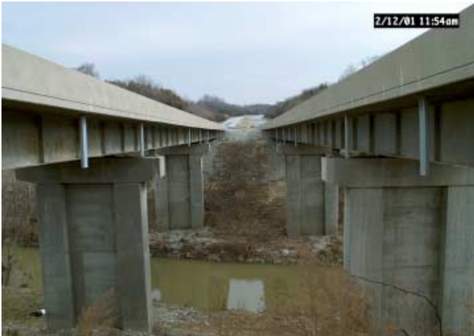
Figure 9. KY 9002 (Bluegrass Parkway) over the Chaplin River in Nelson County prior to painting.
